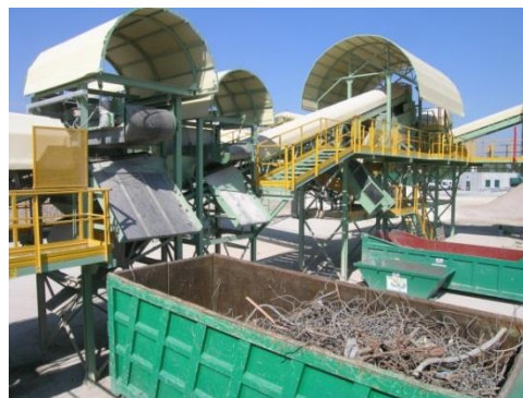
C&D waste recycling plant, Source: ANPAR
