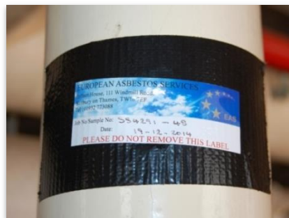
Asbestos marked pipe, Source: UEFG
